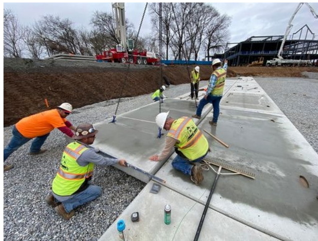
Fig. 10 – Hand guiding a floor slab of a single level system into position
