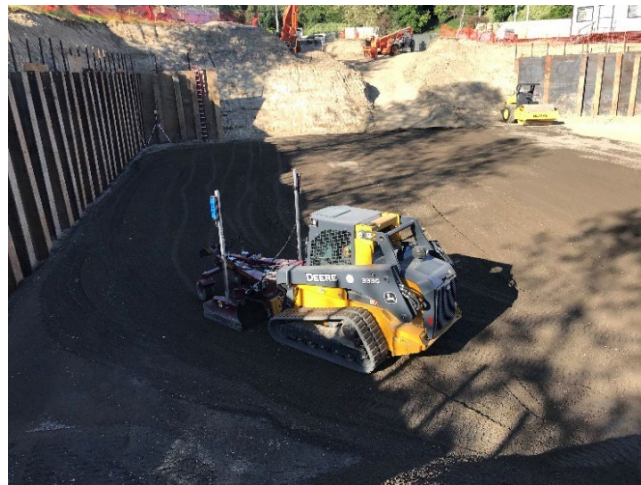
Fig. 2 – Using a skid steer with laser grader to level the base of a large detention system.
